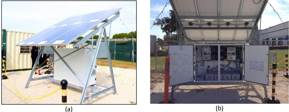
Figure 4. Photovoltaic System installed near the MSTB in order to power the sensor systems during energy analysis. Figure (a) shows the 1040 W PV array and mounting structure. Figure (b) shows the system enclosure with energy conversion, storage, control and remote monitoring modules.
