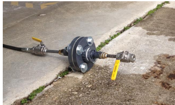
Figure 7. Gasket pressure testing assembly.
