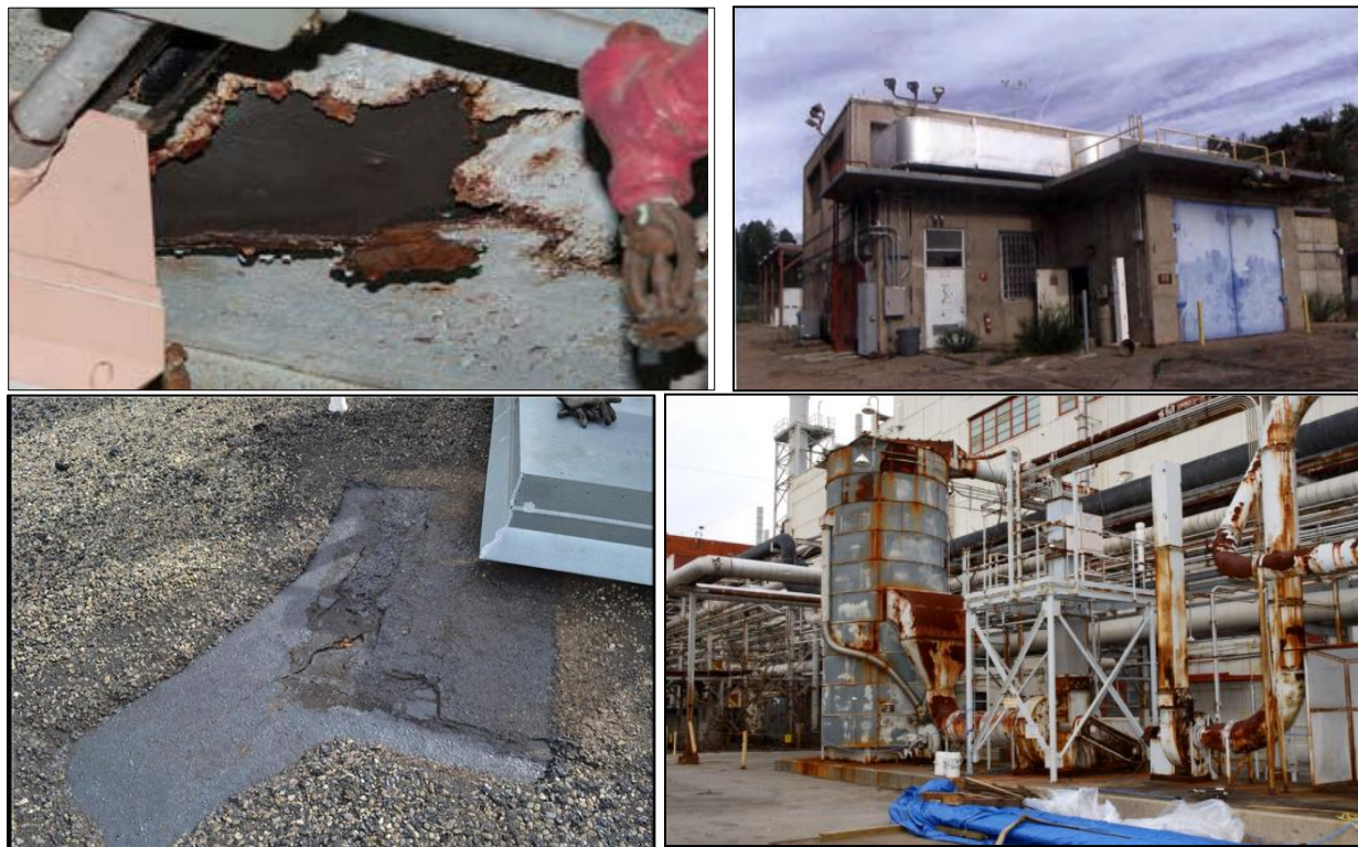
Figure 8. Aging infrastructure at DOE facilities.
