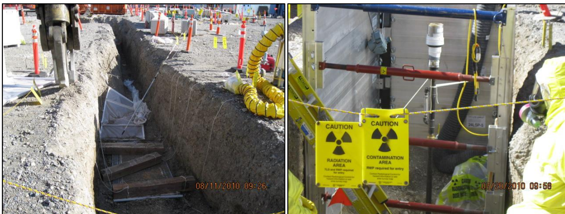
Figure 15. Trench exposing underground piping system(left) and piping system containing contaminated liquids (right).
