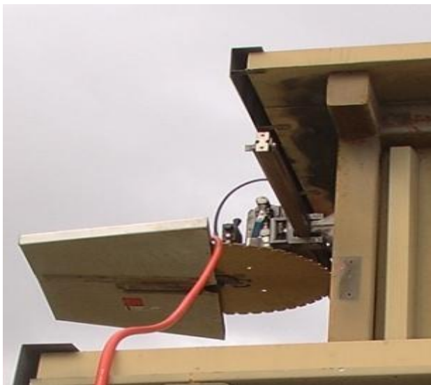
Figure 27. Track mounted wet cutting saw at LLNL.with a diamond blade used at LLNL.
