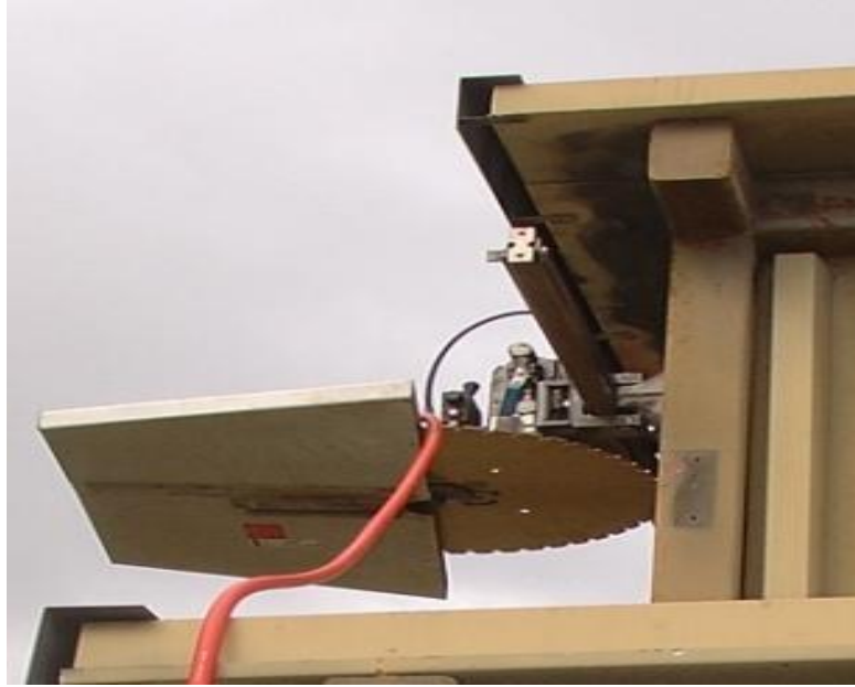
Figure 67. Track mounted wet cutting saw at LLNL.with a diamond blade used at LLNL.
