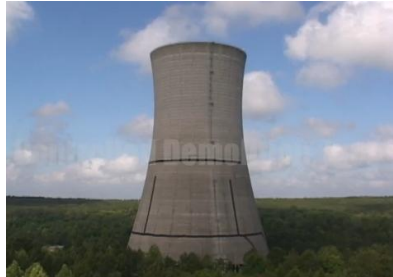
Cooling Tower (before)
