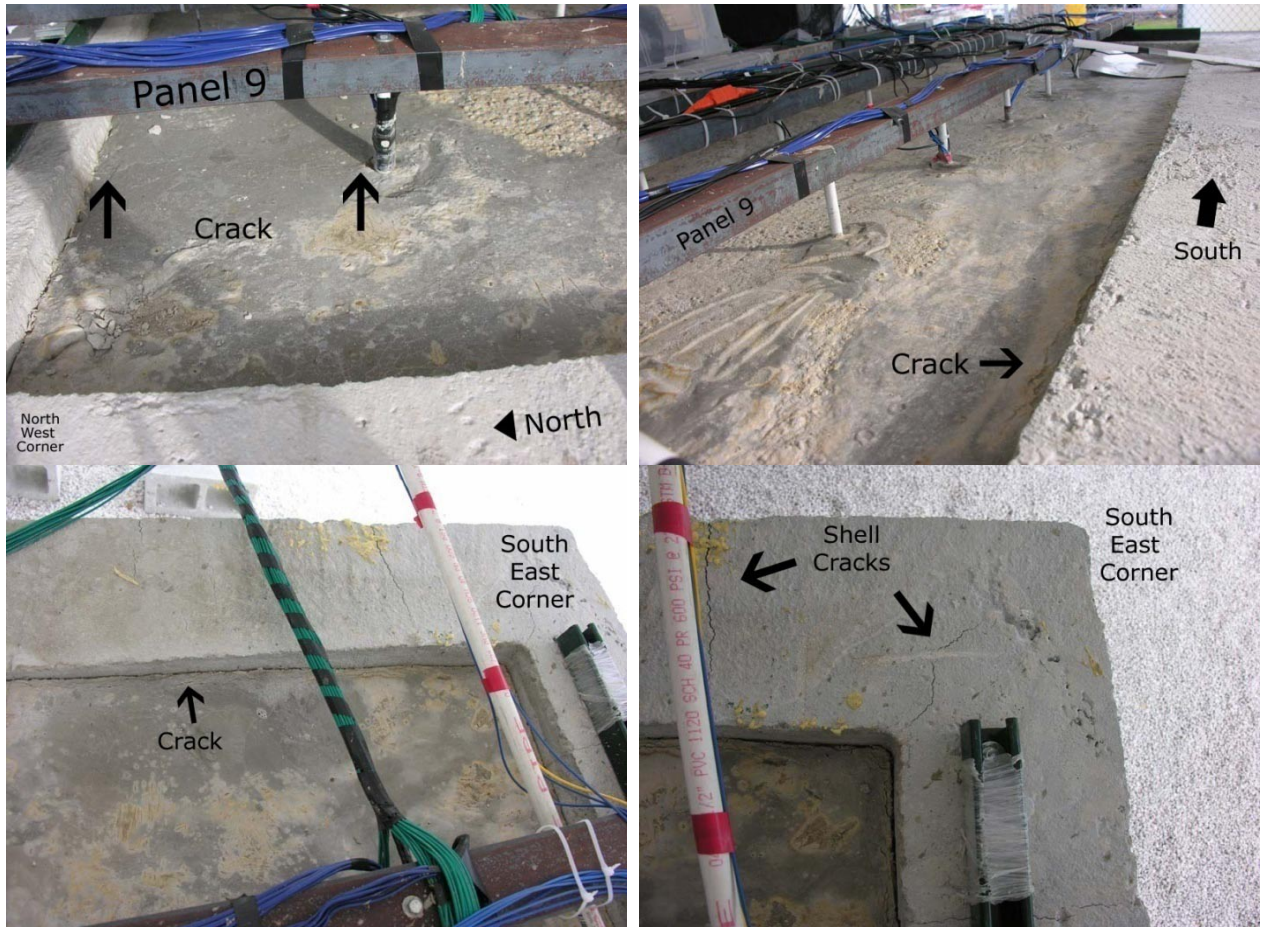
Figure 13. Cracks developing on cube surface.
