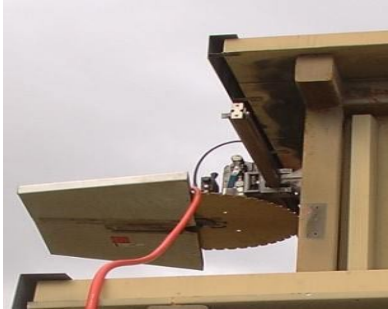
Figure 17. Track mounted wet cutting saw at LLNL with a diamond blade used at LLNL.
