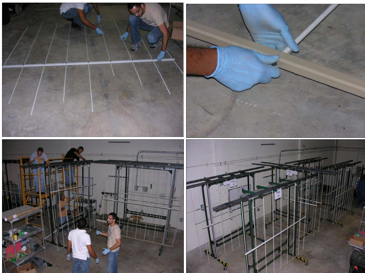
Figure 8. Assembly of the ISDSN sensor frames and sensor racks.
