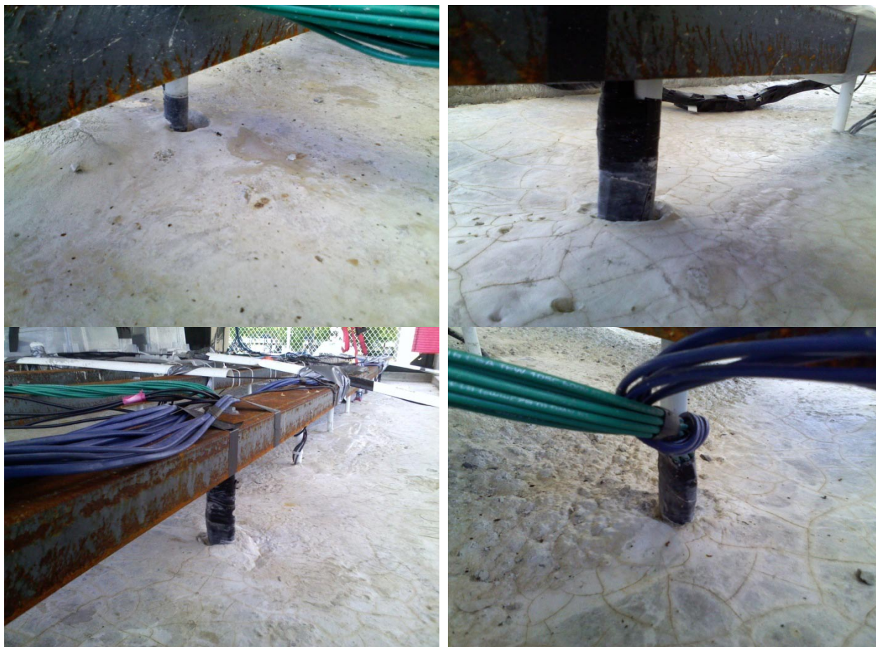
Figure 14. Cavities developing around rods.
