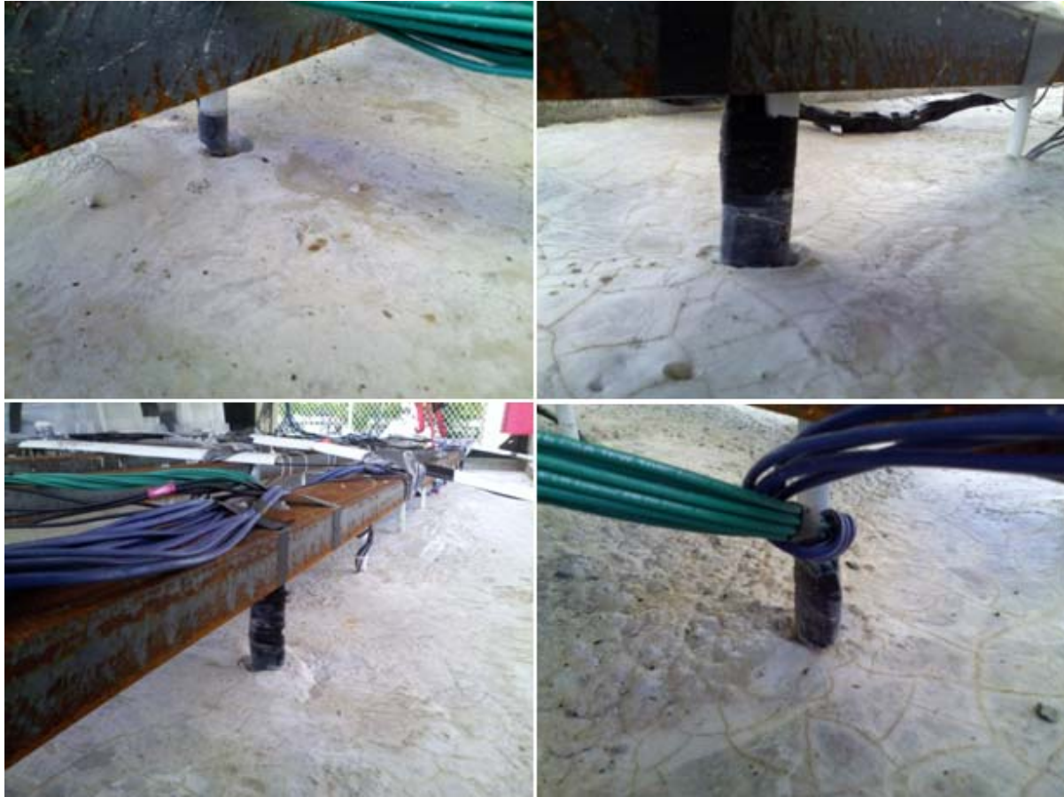
Figure 41. Cavities developing around rods.
