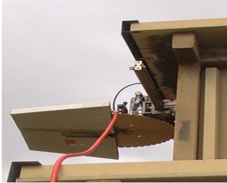
Figure 44. Track mounted wet cutting saw at LLNL with a diamond blade used at LLNL.
