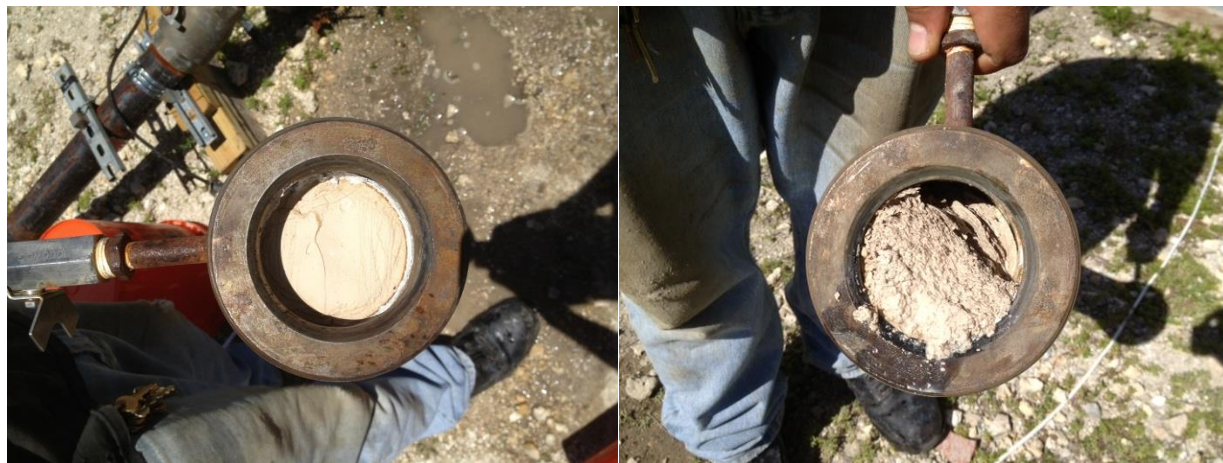
Figure 10. Kaolin-plaster plug before and after unplugging.
