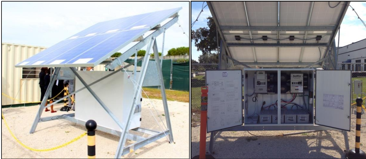
Figure 10. Photovoltaic system in support of ISD test site at FIU.
