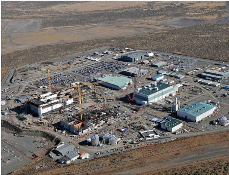
Waste Treatment Plant (WTP) or VIT Plant
