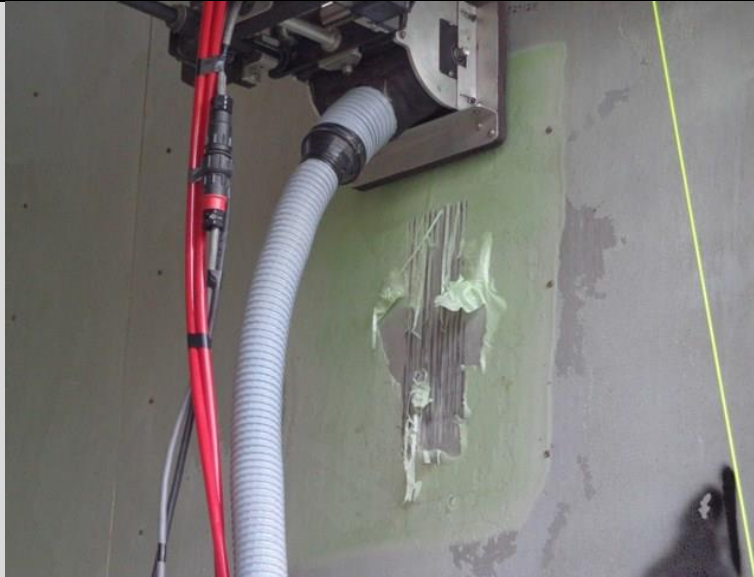
Figure 4-2. ICM remote platform using a brush with a vacuum shroud to remove strippable coating from vertical surface.
