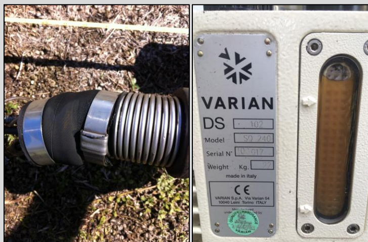
Figure 1-14. Failure of the rear cavity, moisture accumulated in the vacuum pump.
