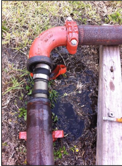
Figure 1-4. Issues encountered after clearing the first elbow.
