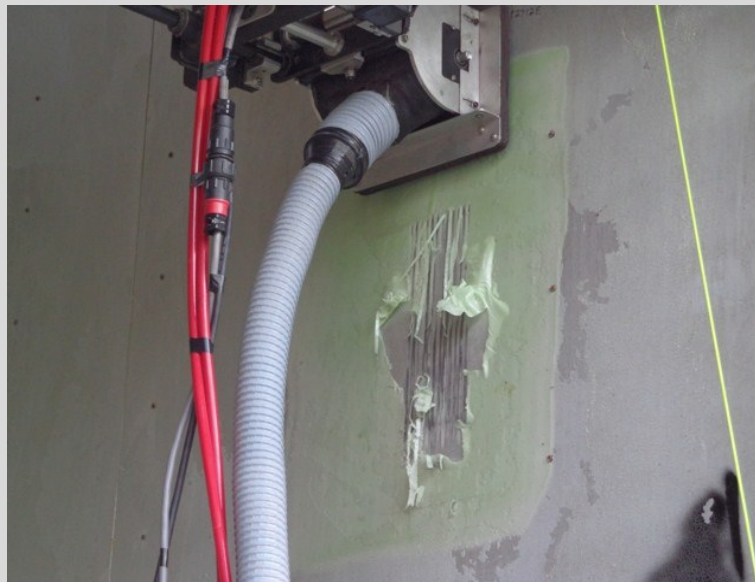
Figure 4-4 ICM remote platform using a brush with a vacuum shroud to remove strippable coating from vertical surface.
