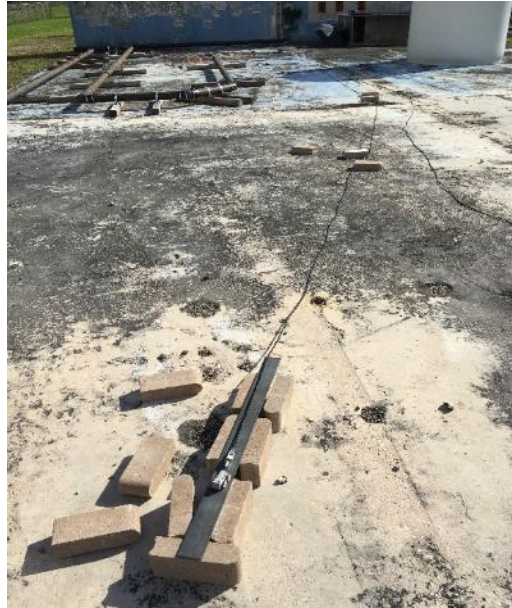
Figure 1-33. Outdoor-test with the mini rover pulling a cable of 50 feet. Two sets of concrete blocks were placed along the cable to simulate the corners along the ventilation channels underneath the tank.
