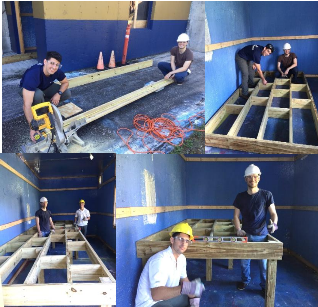
Figure 3-6. Construction begins on selected hot cell mockup design - DOE Fellows constructing raised floor.
