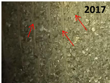
Coarse aggregates and steel rebar exposed (arrows)
