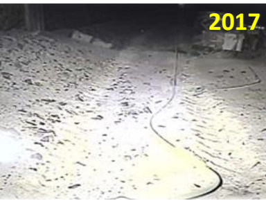
Accumulation of concrete products (e.g. CaCO 3 )
