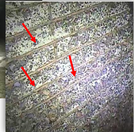
Degraded concrete exposing the steel rebar (red arrows). 1
