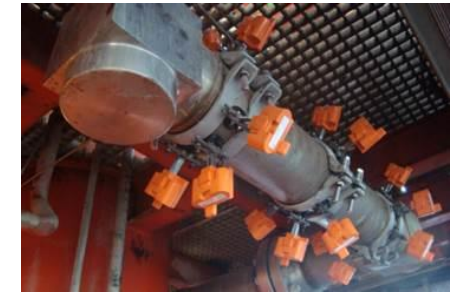
Permasense – guided wave sensors
