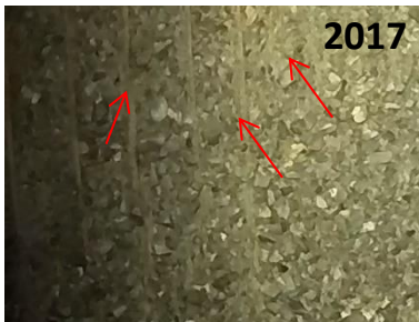
Coarse aggregates and steel rebar exposed (arrows)
