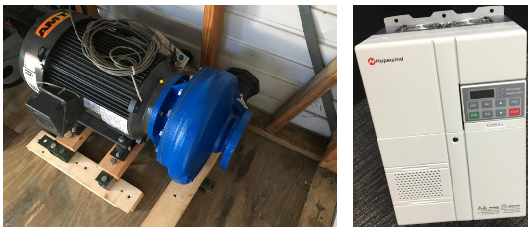
Figure 10. Slurry pump and variable frequency drive for the flushing studies.
