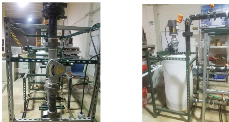
Figure 82. Flow meter [4] (left) and mixer and supporting stand (right).
