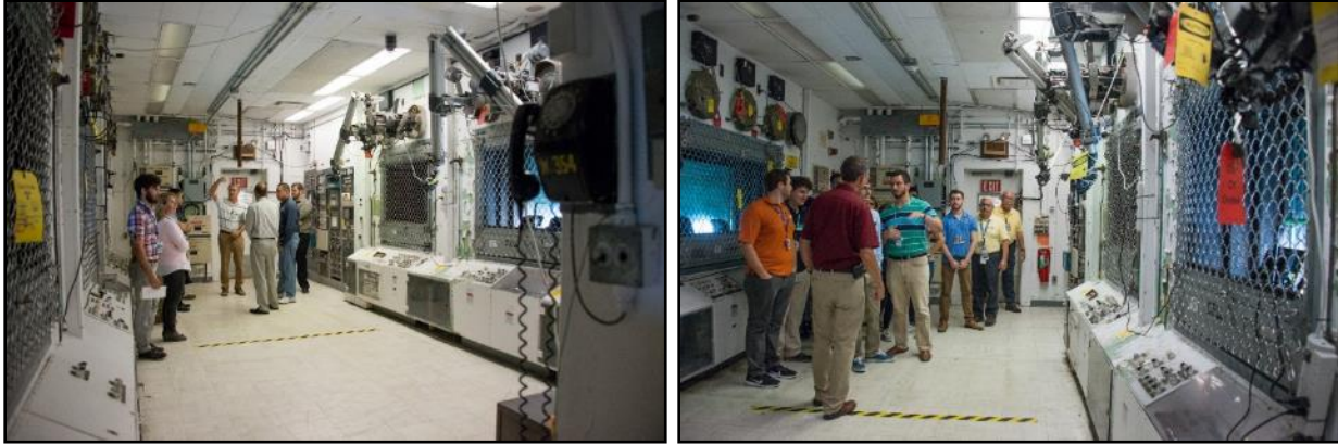
Figure 15. Touring the SRS 235-F Plutonium Fuel Form (PuFF) Facility Operator Station Base.
