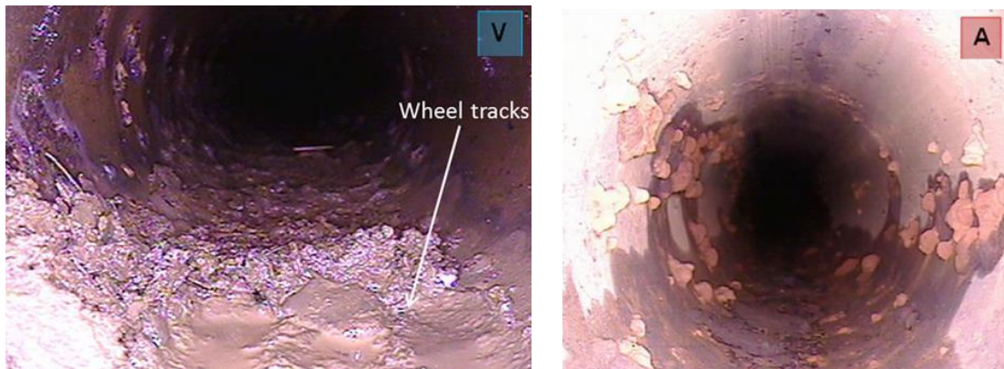
Figure 35. Existing condition of DST’s drain lines (WRPS).
