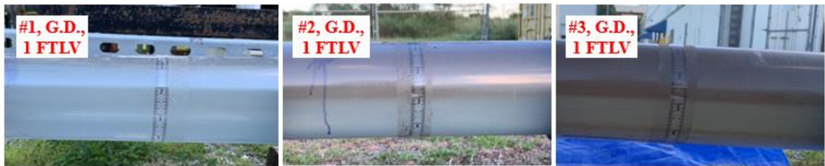
Figure 8. During-flush (up) and post-flush (bottom) assessments gravity-drained pipeline with target FTLV of 1.
