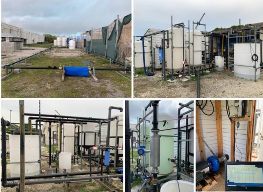
Figure 3. Pipeline constructed for flushing experiments.
