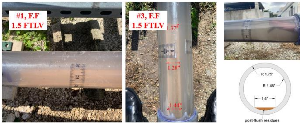
Figure 6. Post-flush conditions of loop at start and end point clear sections one-day after flushing.
