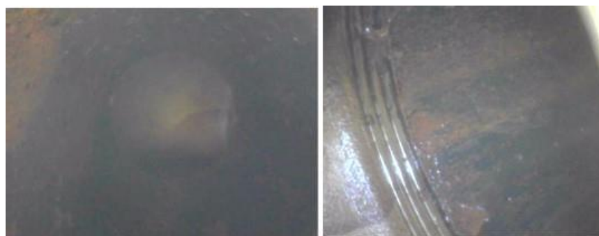
Figure 108. Pipe surface – internal 3-inch section (left) and eroded, corroded pipe threads (right).
