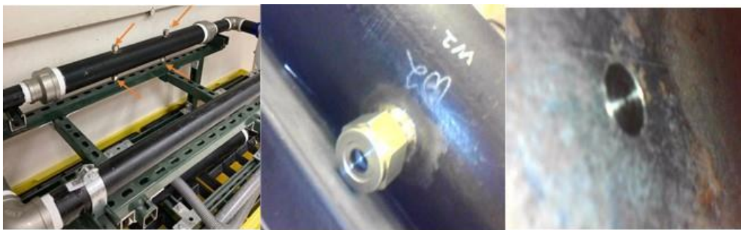
Figure 101. Coupon locations (arrows) (left), coupon joint (center) and borescope image of the coupon (right) in the pipe loop.
