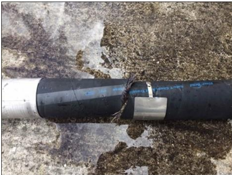
Figure 125. A rupture hose failure.
