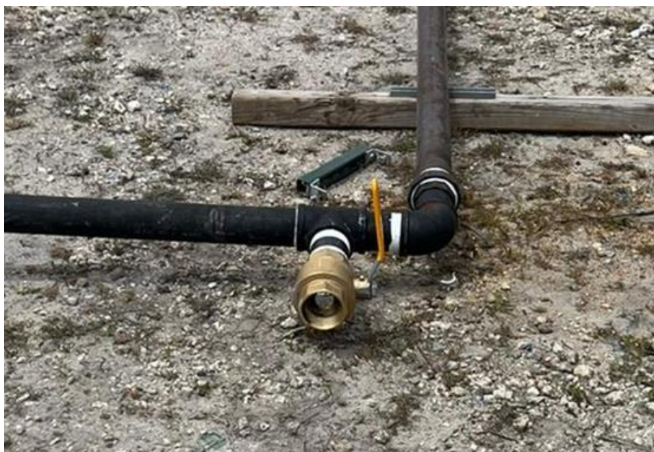
Figure 5. Gravity drained discharge valve at the 90-degree section of the flushing loop.
