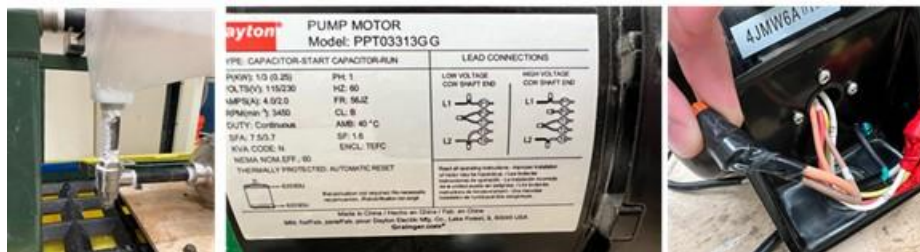
Figure 109. Chemical precipitates (left), pump wiring configuration (center) and new wiring (right).
