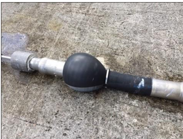
Figure 126. Internal hose failure.
