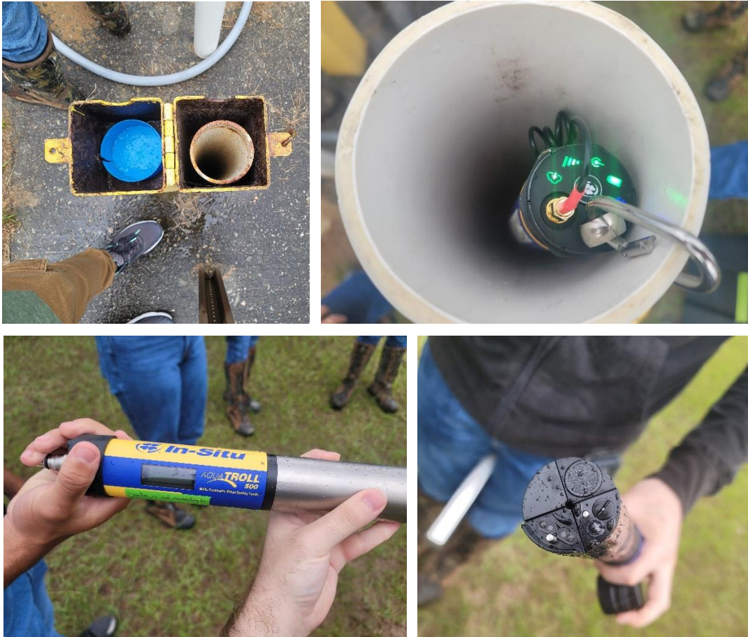
Figure 19. SRS monitoring well, sensors and data collection system used to obtain groundwater monitoring well data.
