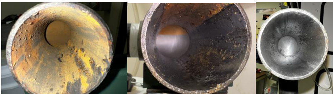
Figure 101. Chemical corrosion from Phase I testing (left and center) and clean pipe component (right).
