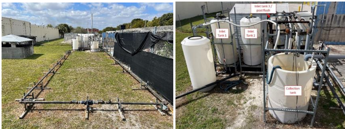
Figure 3. Experimental flushing pipe loop with storage and flushing tanks.
