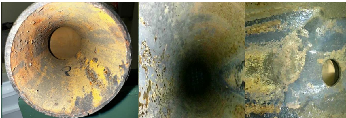
Figure 98. Borescope images of corroded internal structure of the pipe loop.
