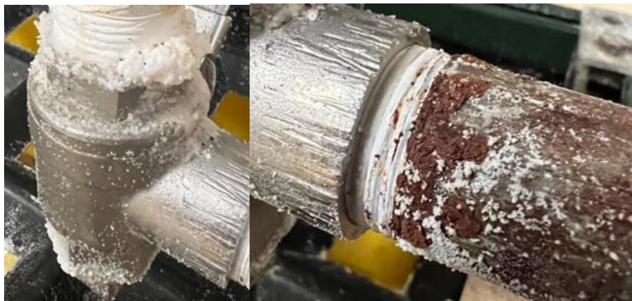
Figure 107. External minor leakage salt formalization and rust deterioration.
