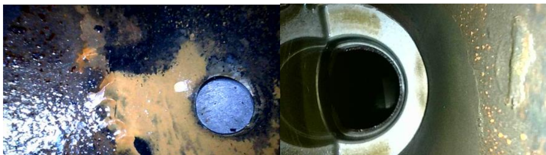
Figure 105. Wall damage near Coupon 4 hole (left) and wall damage with chemical solution in pipes (right).
