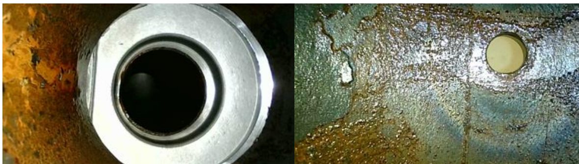
Figure 104. Pipe wall damage near the expander (left) and wall damage and Coupon 1 hole (right).
